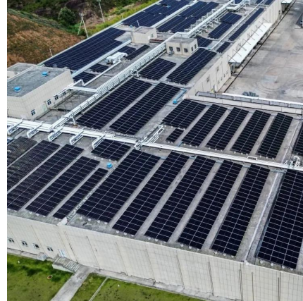
80kW Off Grid solar system (115.2kWh)
