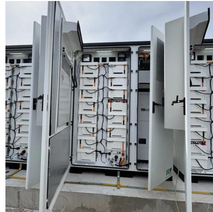
Containerized Battery Energy Storage Systems (BESS)
