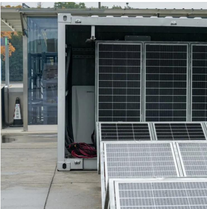
Battery energy storage system (BESS)...
