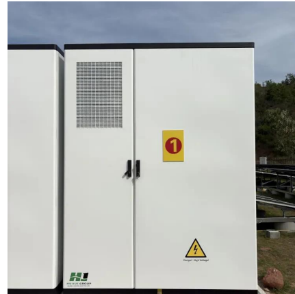
20FT Container 250KW 803KWH Battery ...
