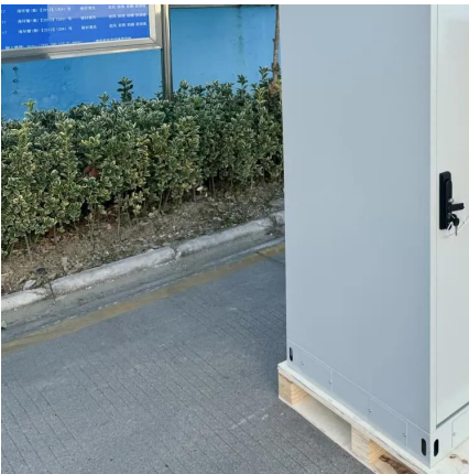
Sunway 1Mw Battery Container Energy Storage System
