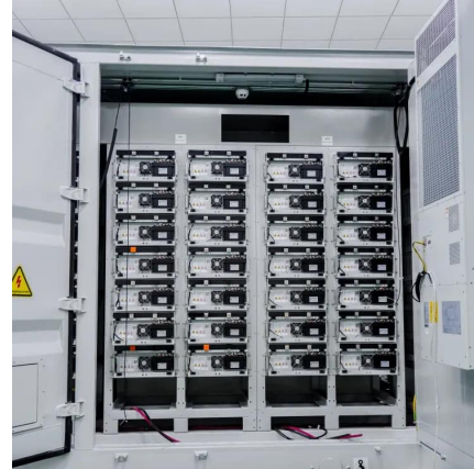
2MWH Containerized Solar Battery Storage System
