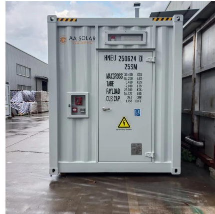
Ess Energy Storage Container
