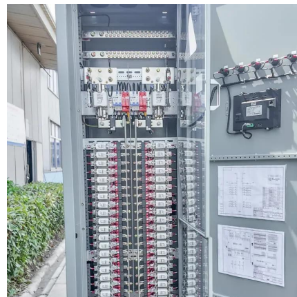
Energy Storage Container & BESS Container ...
