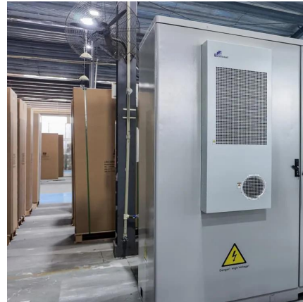
Outdoor Base Station Cabinet
