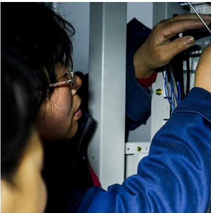
Mobile communication base station
