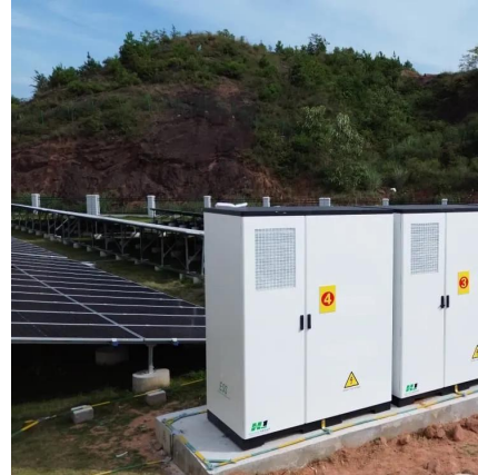
Energy Storage Enclosures/Cabinets
