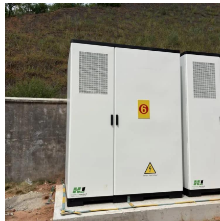
Solar Container , Large Mobile Solar Power ...
