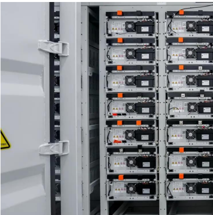
Communication base station inverter provided by North Korea
