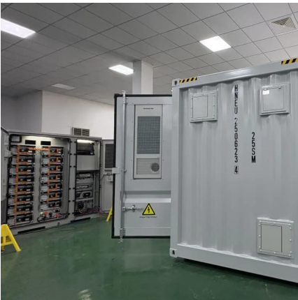
containerized battery storage , SUNTON POWER
