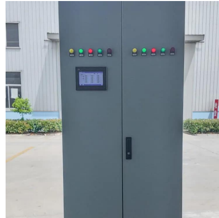
containerized battery storage , SUNTON ...
