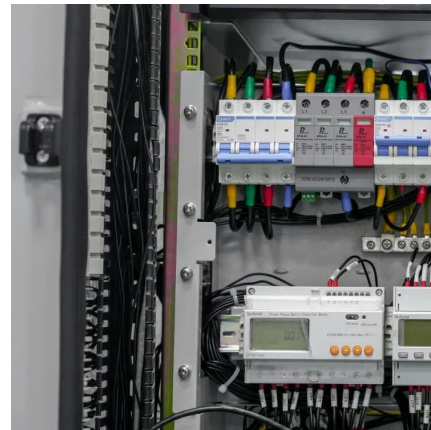
containerized battery storage , SUNTON POWER
