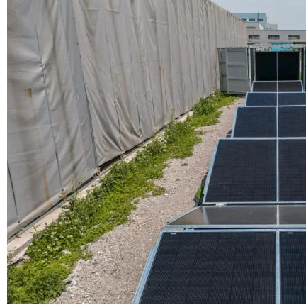
Containerized energy storage , Microgreen.ca
