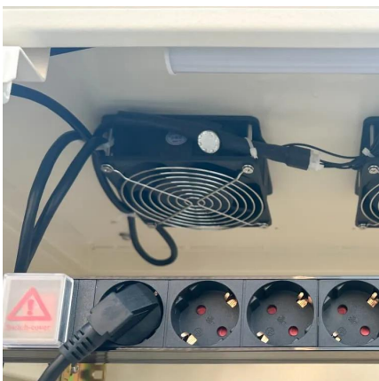
30 kW String Inverters
