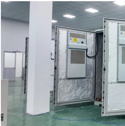
30000 Watt DC Solar Inverters
