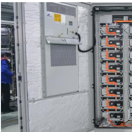
Outdoor Integrated Energy Storage Cabinet_On And
