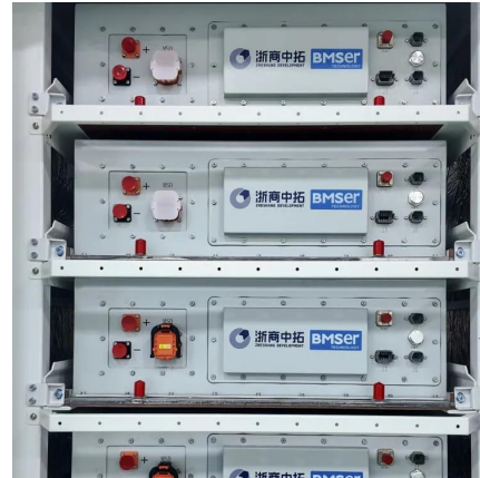
On-site rooftop solar at data centers: ...
