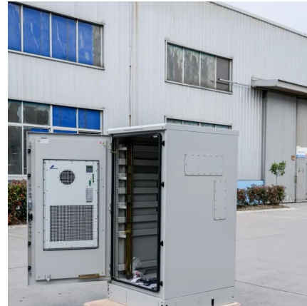
Alxa Solar Energy Storage Project, Inner Mongolia
