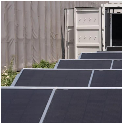
South tarawa energy storage
