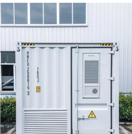
Site Support Cabinets , SS Cabinets , Power ...
