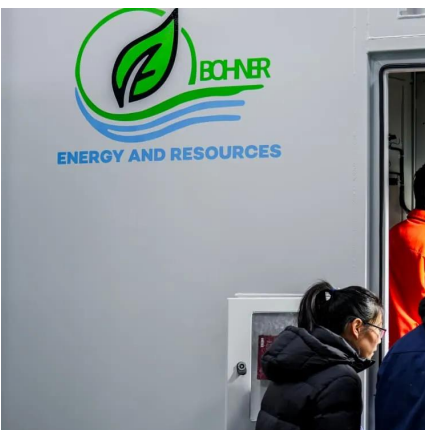
20FT Container 250KW 803KWH Battery ...
