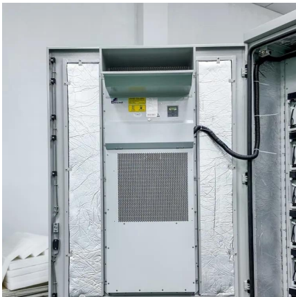
200kwh LiFePO4 Battery Container for PV Solar Energy...
