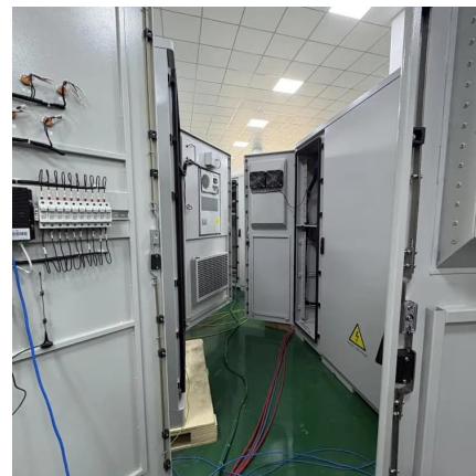
Photovoltaic energy storage container
