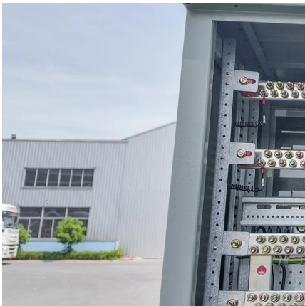
Communication container station energy ....
