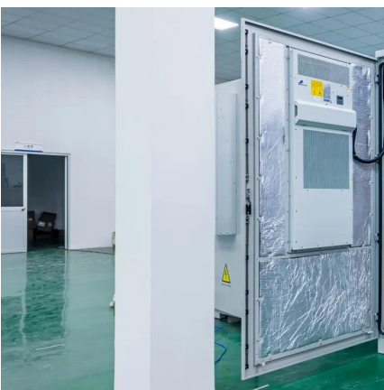
TRIPOLI ENERGY STORAGE PROJECT
