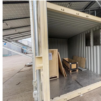
Container Energy Storage System on Grid ...
