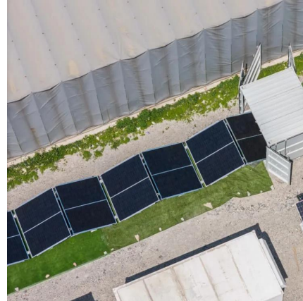
Deployment of 250kW/600kWh Industrial ...
