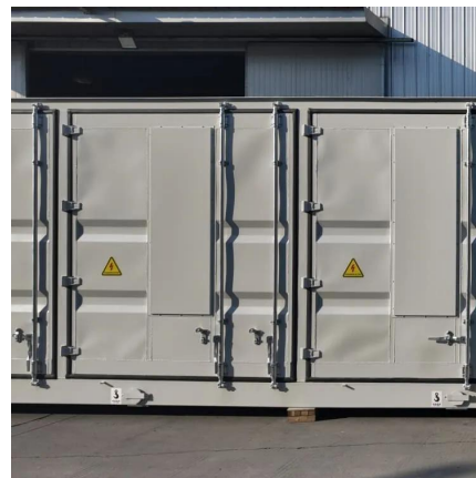
Ukraine 400kWh Energy Storage Cabinet Project
