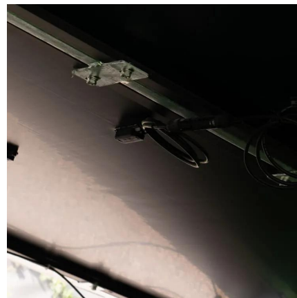
How a Containerized Battery Energy Storage System Can ...
